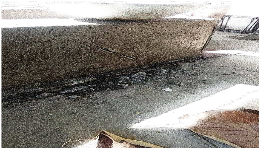
Fig. 4: Preformed crack beam.
